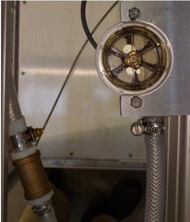
Figure 13: Coolant Flow and Temperature Sensors
